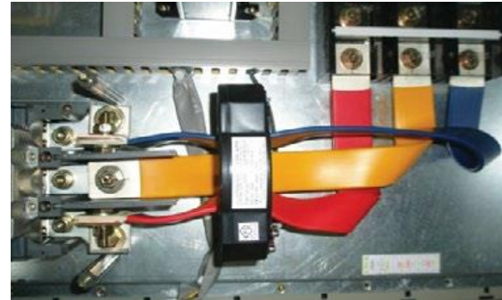
▲ Current Transformer (CT)
