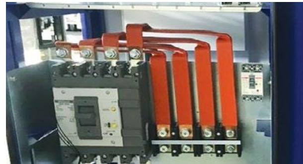
▲ P-Company Battery Charger
